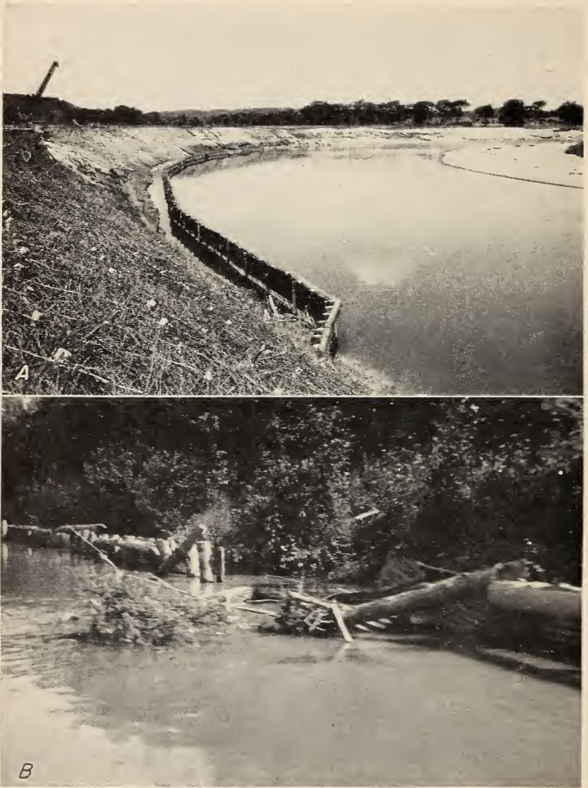
FIGURE 7.—Revetment of log piling and corrugated metal. A , Retaining wall, with bank sloping, planting, and brush matting in various stages of completion, 1938; B , section of revetment destroyed by the impact of floods as photographed in 1945.
